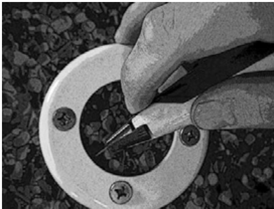
Trim liner from return opening.
