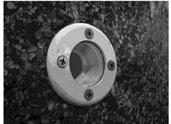
Return faceplate installed.
